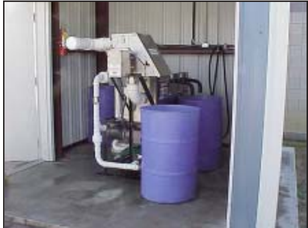
SuperCeptor® S-2750 Installed In Calhoun State Prison, Morgan, GA
