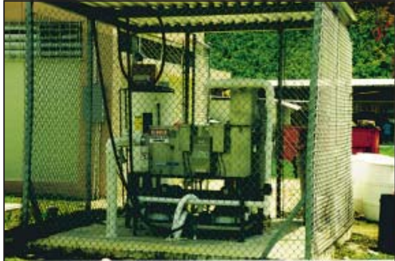
Pictured is one of two Big Dipper® SuperCeptor® grease/water separator systems located at the Sabana Hoyos Correction Institution and Sabana Penal Camp in Puerto Rico. The units are in an outdoor location for pretreatment of kitchen water.
